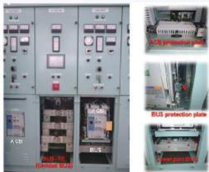
Marine Power Distribution Panel
