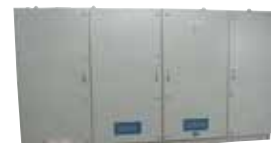
ESDS Control Panel
