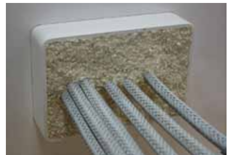
Apply NF-23 so as not to leave any space, especially around any of the cables.
